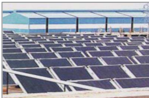
Fig 3.17: Solar Panels to trap solar energy
